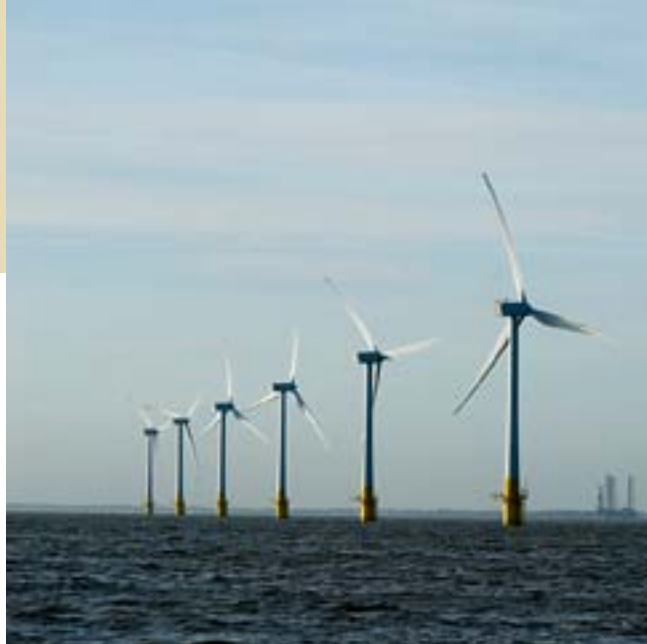
Burbo Bank, Liverpool Bay, UK © RenewableUK
