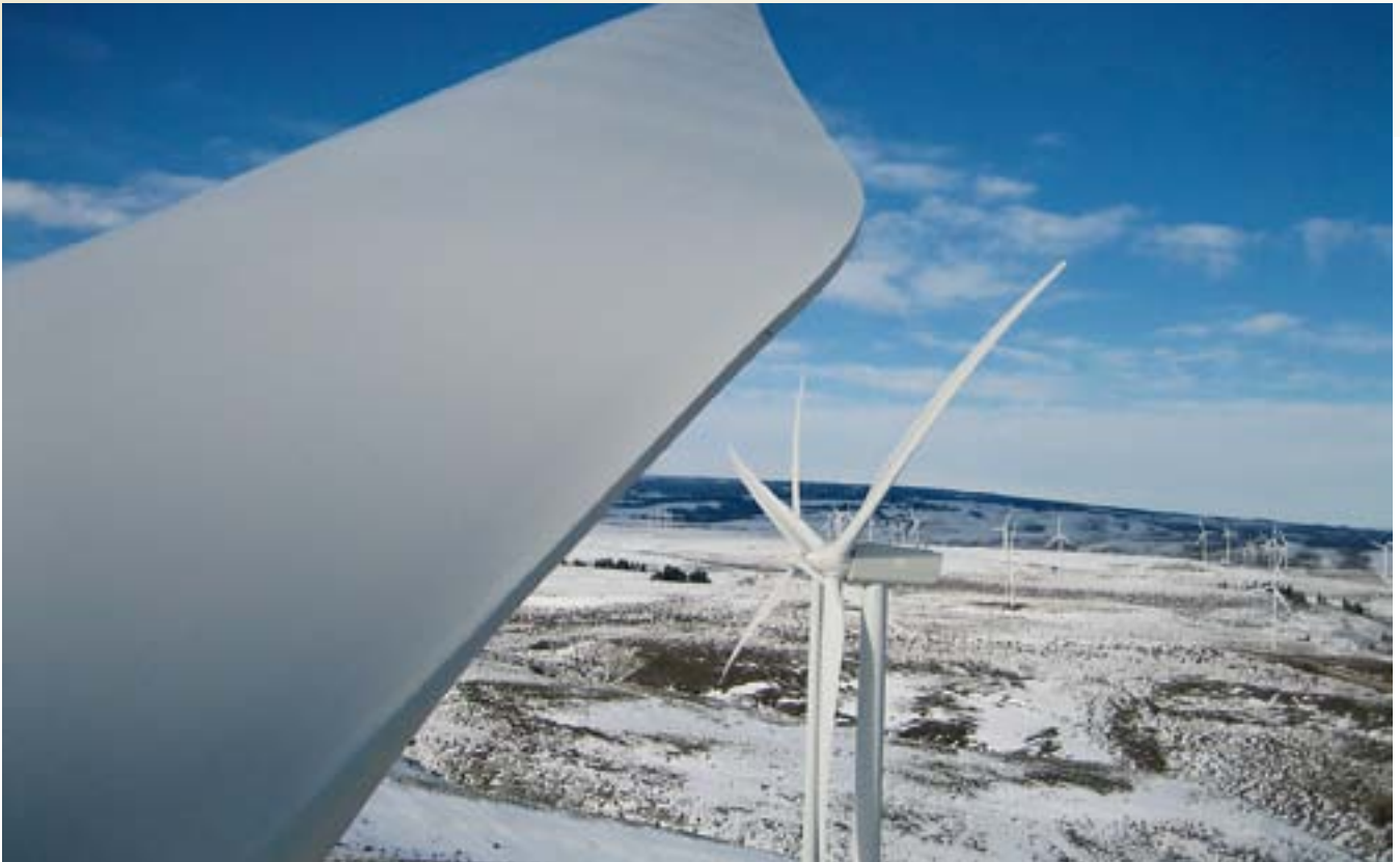
Wild Horse Wind Power Project, Kittitas County, Washington state. Total generating capacity 228.60 MW © American Wind Energy Association (AWEA)
