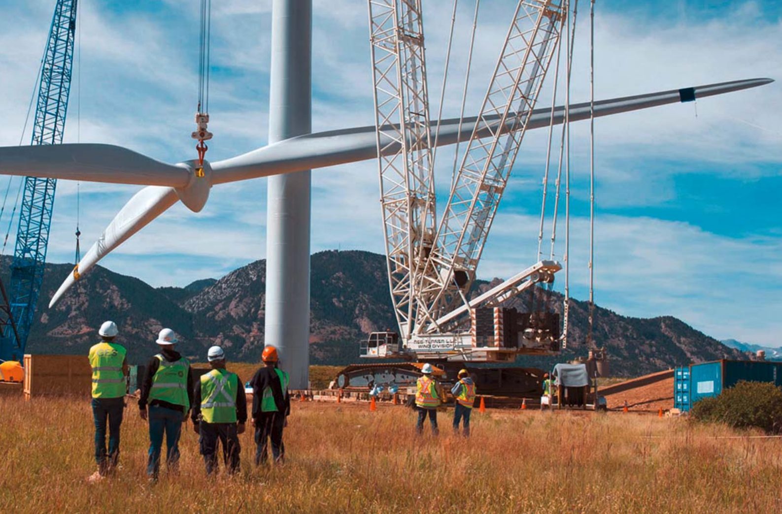
Construction of a wind turbine in Ngong Hills, Kenya © Construction Review Online
